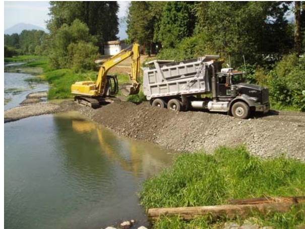
Gravel being hauled to the site and an access road being created along the stream edge
