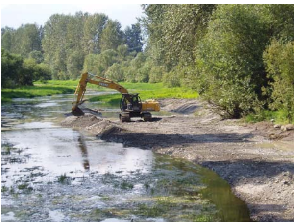
A berm being constructed along the edge of the spawning channel to create the appropriate flow conditions over the spawning gravel
